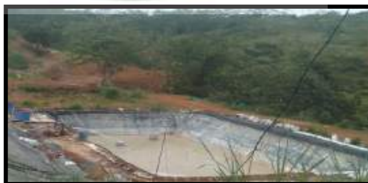
Sumber : Pengolahan Emas PT. Golden Pricindo Indah Gambar 2.8 Water Barrier Pond
